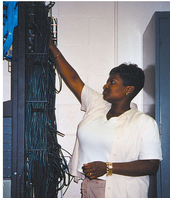
► The huge jumble of wires is incomprehensible to most people, but Aleatha knows exactly where each one goes.
